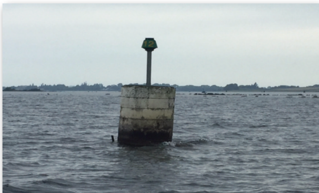
Photograph No. 2: Marker No. 112 showing a partially underwater metal bar from a previous navigation marking.
